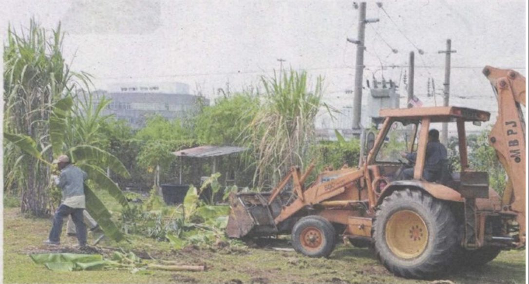
Council workers clearing the sugarcane and banana plants on KTM reserve land.
